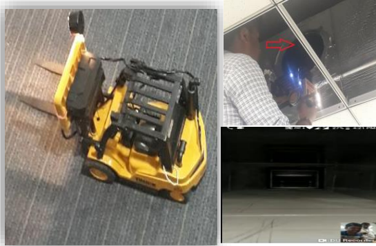
Remote Controlled equipment for HVAC ducts
