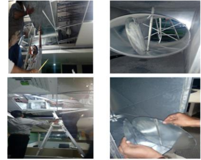
VAV Services by In-house team
