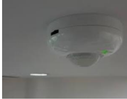
Motion Sensors for ODC and switch room lighting control
